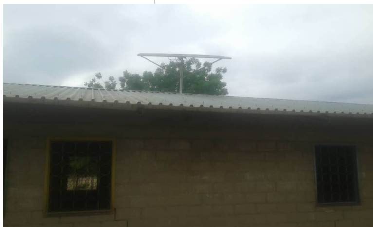
PV system installed at Ndawera Primary school
