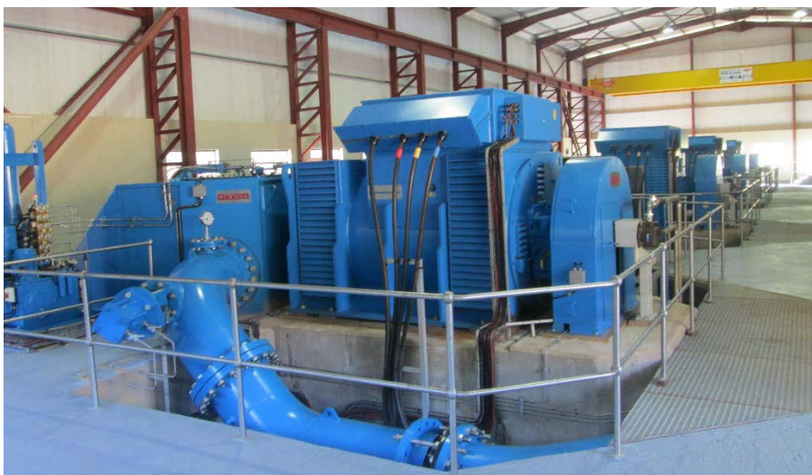
Fig. 3 - Visit of the run-off-river hydro power station (generator house)
